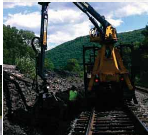
Dave Hutton working with PT-1 to install roughly 2000' of power cable at a new interlocking location "Coal" at Glen Onoko in Jim Thorpe.
