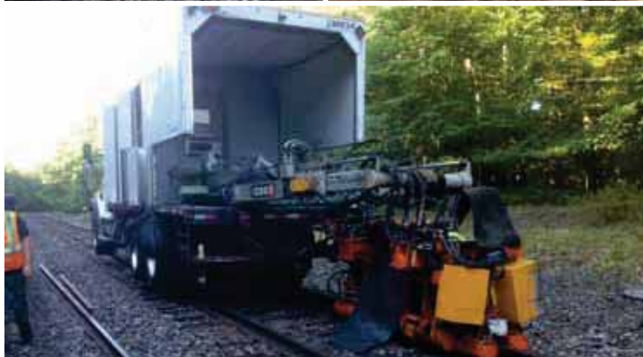
The flash butt welding truck with the welding unit setting up a weld on #2 track. Frank Sebelin takes the picture of the work being completed by GWPeoples.
