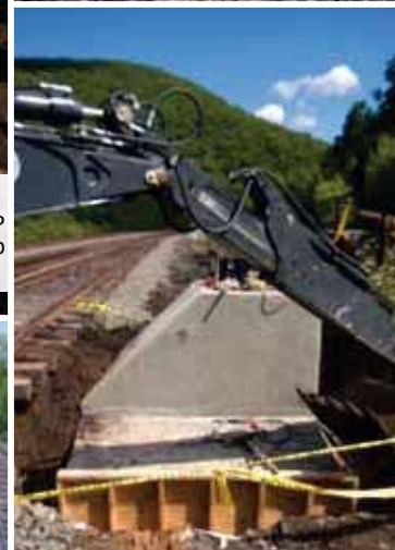
Final stages of clean up and backfill around a newly constructed cantilever base at MP 124.77 Coal to install a new signal.
