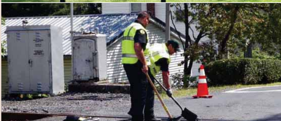
Beckville Rd. RR Crossing Lt. Johnson and Officer Fredmski make cold patch repairs to pot holes.
