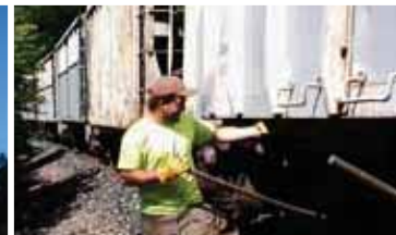
Josh Rodney dumping ballast, with the assistance of the work train provided by operations, on the shoulders of #1 track between MP 166 – 164.1.
