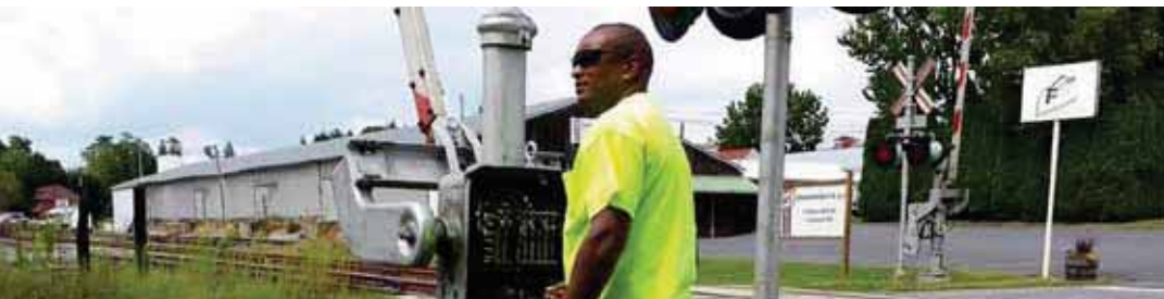
Darnell Young completing a federally mandated monthly crossing test at Wall Street in Leesport, Pennsylvania.
