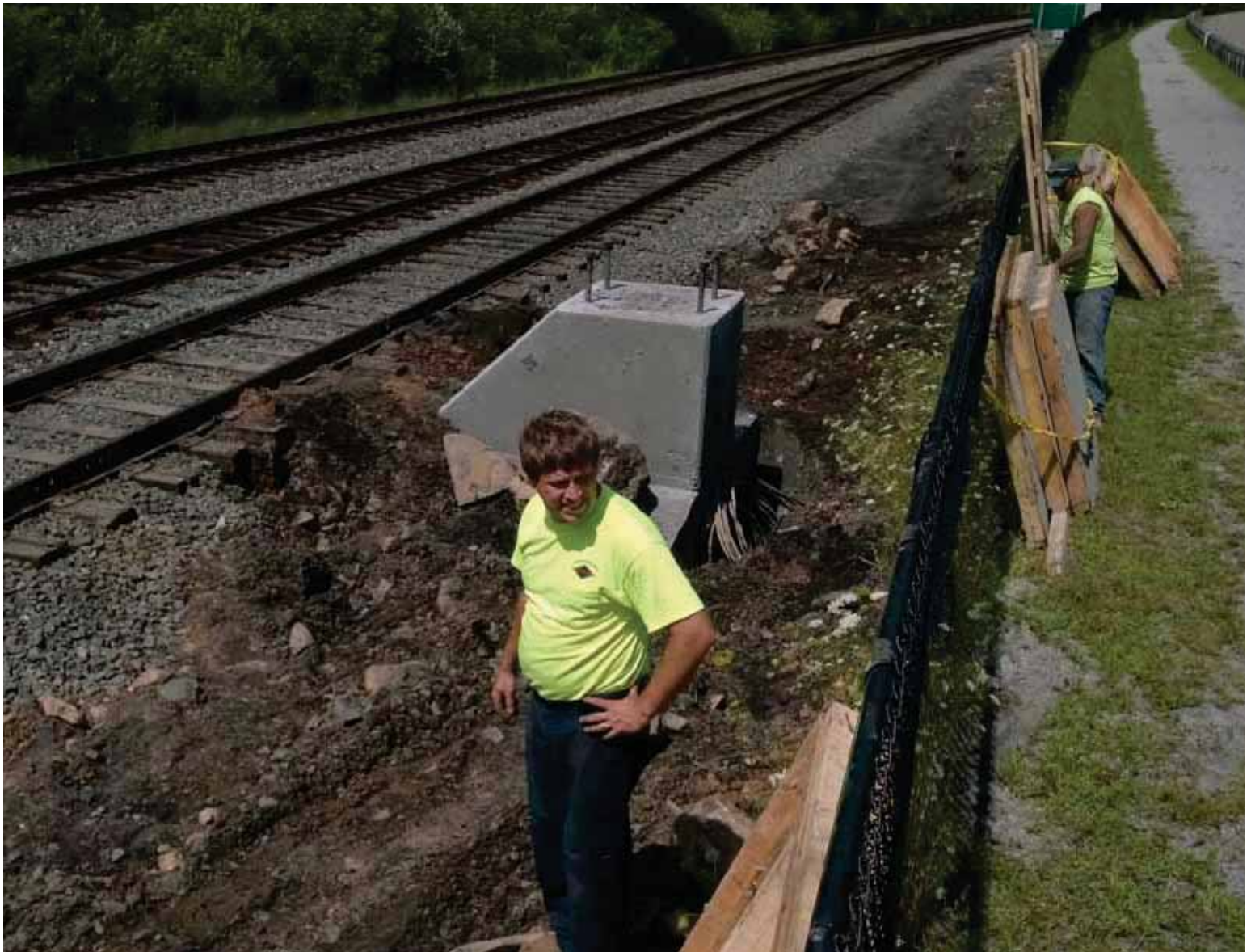
Jonathan Barket at the future site of Coal Interlocking plotting the next move with Mario DeMarco working in the background.
