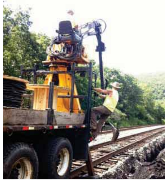
Dave Hutton working with PT-1 installing roughly 2000' of power cable at a new interlocking location "Coal" at Glen Onoko in Jim Thorpe.
