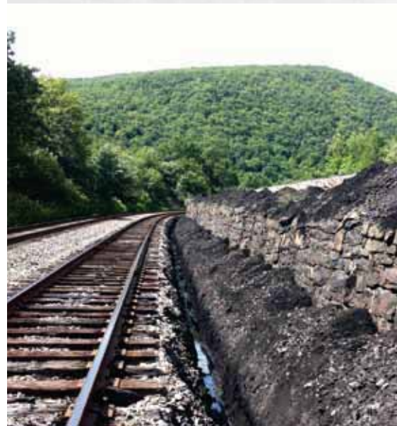
2000' of power cable installed and awaiting backfill at a new interlocking location "Coal" at Glen Onoko in Jim Thorpe.
