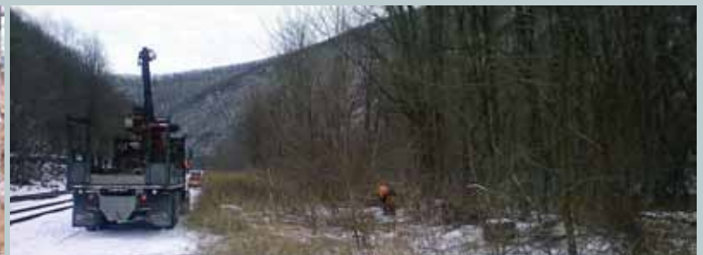
Working with Norfolk Southern along RBMN Lehighton Branch to remove an inactive pole line. Photo by RBMN Signal Maintainer David Hutton.
