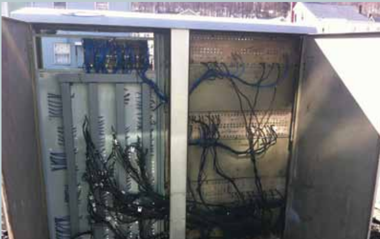
Vine St. Tamaqua crossing rehab complete with new terminal board and relays. Photo by Matt Collins.
