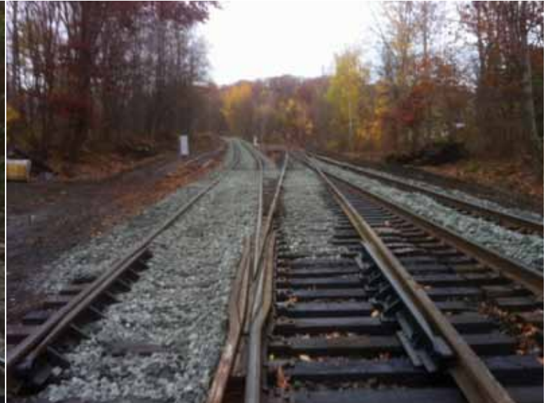
Both frogs, switch points, guardrails, and closure rails installed and ballast dumped, facing north. Photo by Duane Engle.
