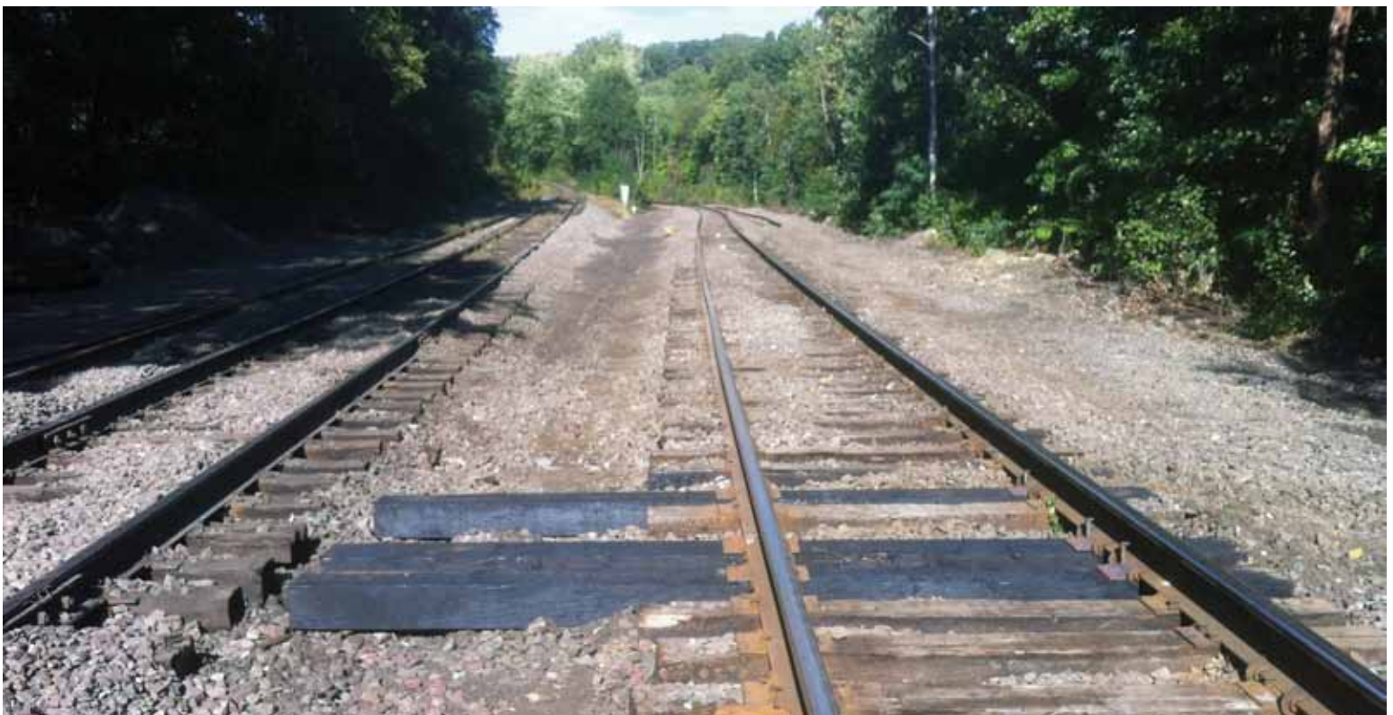
First of three switch timbers installed, facing north. Photo by Duane Engle.
