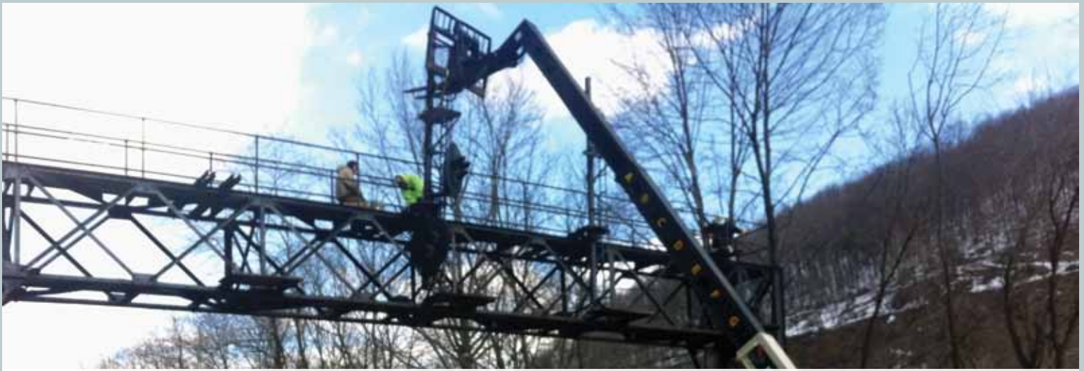
Working alongside of car shop personnel, removing the nearly decade old signal at Pottsville Jct. for rehab work. Photo by Jonathan Barket.
