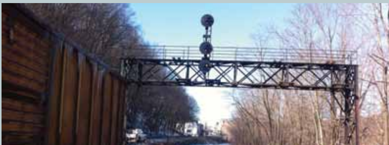
Pottsville Jct. Signal complete and working. Photo by Jonathan Barket.
