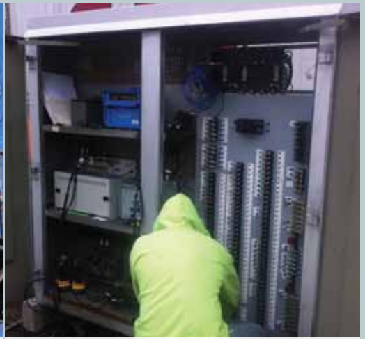
Vine St., Tamaqua crossing receiving a new terminal board and relays. Maintainer Matt Collins begins to make final connections. Photo by Jonathan Barket.
