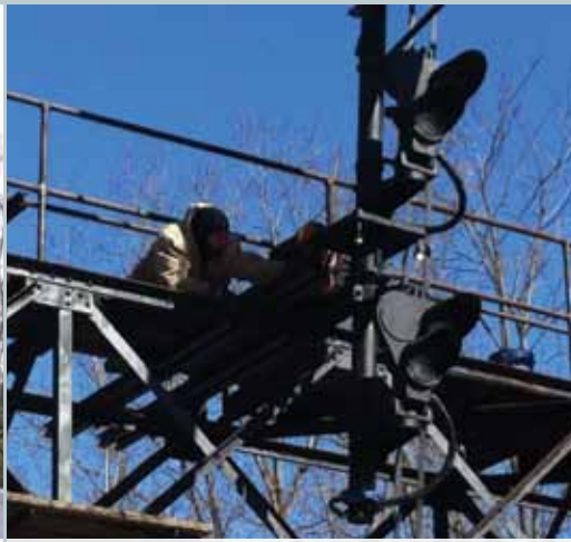
Reinstallation of newly refurbished signal for Pottsville Jct. Maintainers Edward Kopeck and Matt Collins line up bolts to re-secure signal. Photo by Jonathan Barket.
