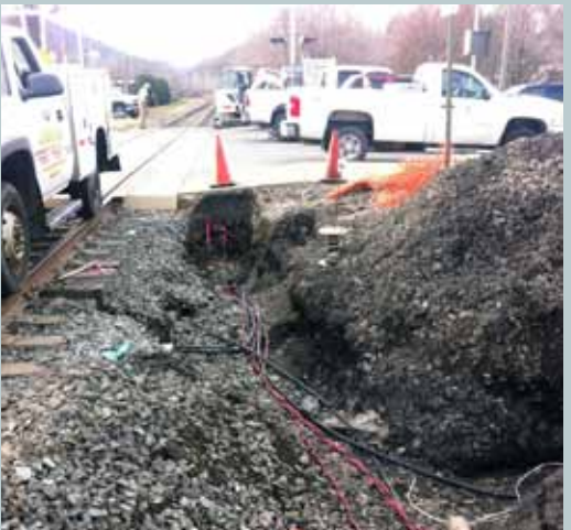
Cable Installation at Bridge St., Tunkhannock to allow for non-interruption of vehicular traffic while trains shift the new facility for D&I Silica. Photo by Matt Collins.
