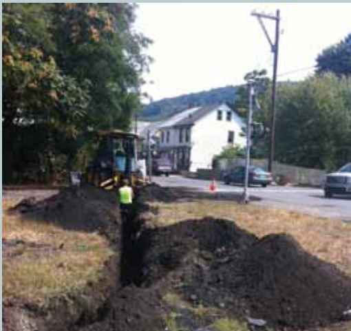
Dave Hutton installing cable at Spruce St., Tamaqua, to enable better warning times to vehicular traffic of approaching trains. Photo by Matt Collins.
