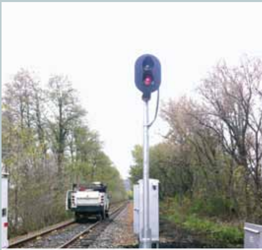
Crossing Indication signal installed and working at Bridge St., Tunkannock for new D&I Silica facility. Photo by Matt Collins.
