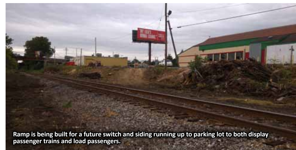
Tracks being constructed at the end of our Tremont Running Track to service Koppys, our new customer.
