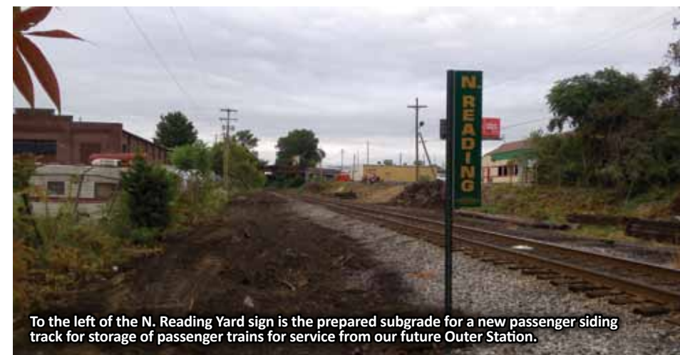
Ramp is being built for a future switch and siding running up to parking lot to both display passenger trains and load passengers.
