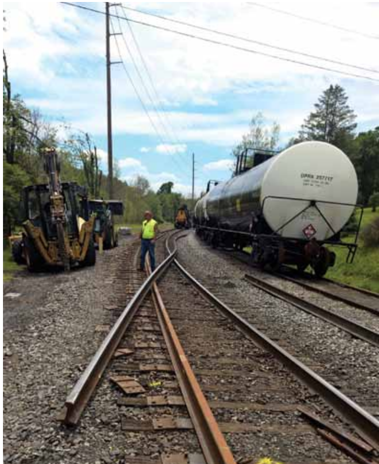
Working on the Reading ML at MP 96.5, crews begin to push the last bit of old rail so the new rail can be spiked into place.
