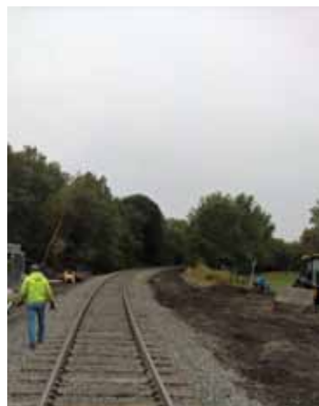
New surfaced curve on Susquehanna Branch looking south from Foote Ave MP 1.91.
