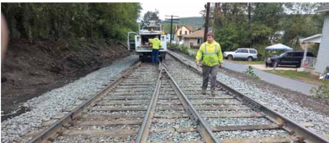
New location of Duryea Jct switch on Susquehanna Branch MP 1.92 north side of Foote Ave crossing. Jonathan Barket checking all the signal components for the new gates and flashers installed at this location.
