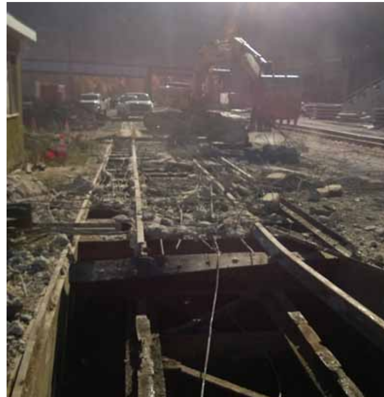
Using an excavator to pull out the rotten old scale so the pit is exposed for fill, the project is well under way to restore use of the runaround track in Jim Thorpe yard.
