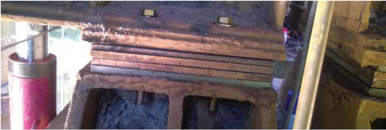
Newly installed shims bolted into place proved the proper elevation to the bridge beams and Susquehanna Branch above.
