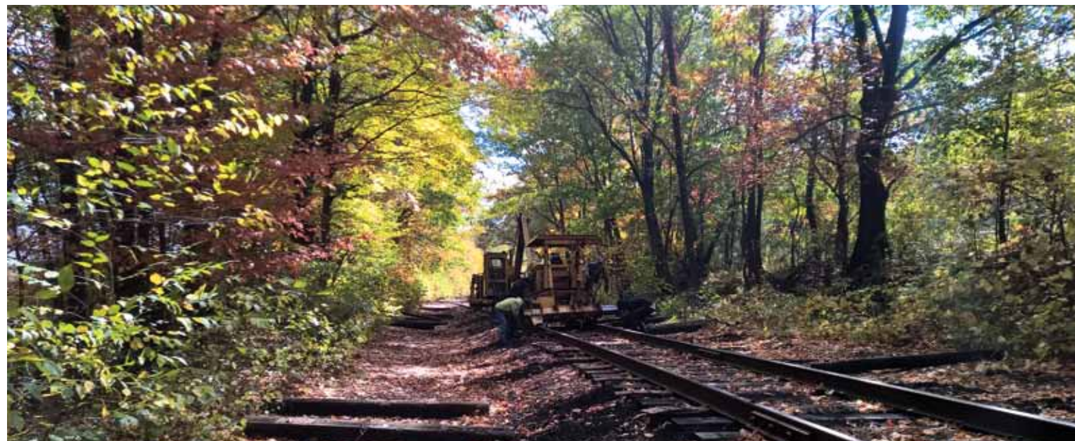
W. E. Yoder tie gang installing ties on Hazleton Line north of Delano Road crossing in Tamanend MP 106.68.
