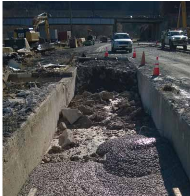
Working with local contractor on site to fill in material into the old scale pit so the track can be reinstalled in Jim Thorpe yard.
