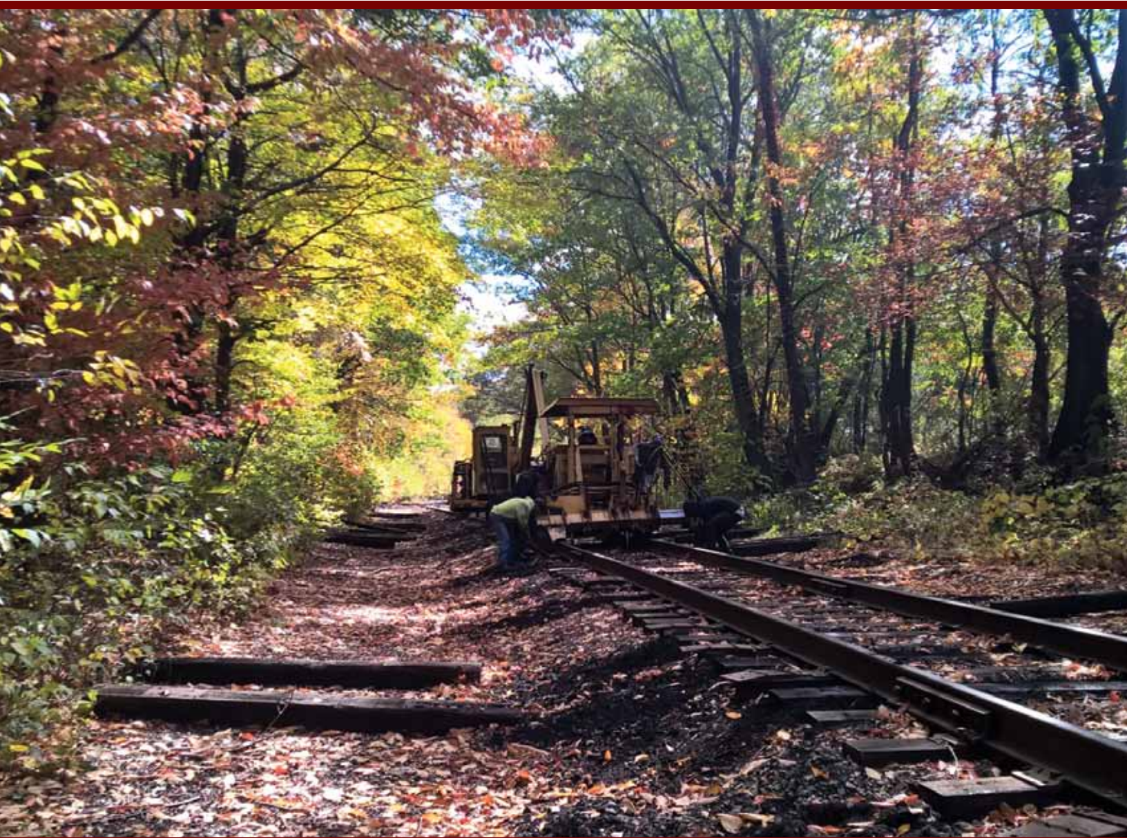
W. E. Yoder tie gang installing ties on Hazleton Line north of Delano Road crossing in Tamanend MP 106.68.
