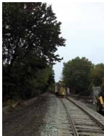
The Dunmore RT MP 0.01 at Foote Ave regulated after the track was realigned to match the relocation of the Duryea Jct switch.
