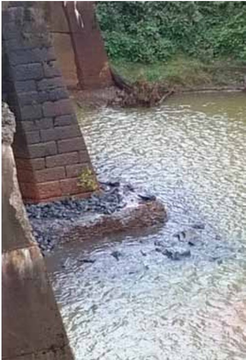
Installing rip rap around the center pier to prevent pier undermining during times of flooding on the Lackawanna River Bridge.
