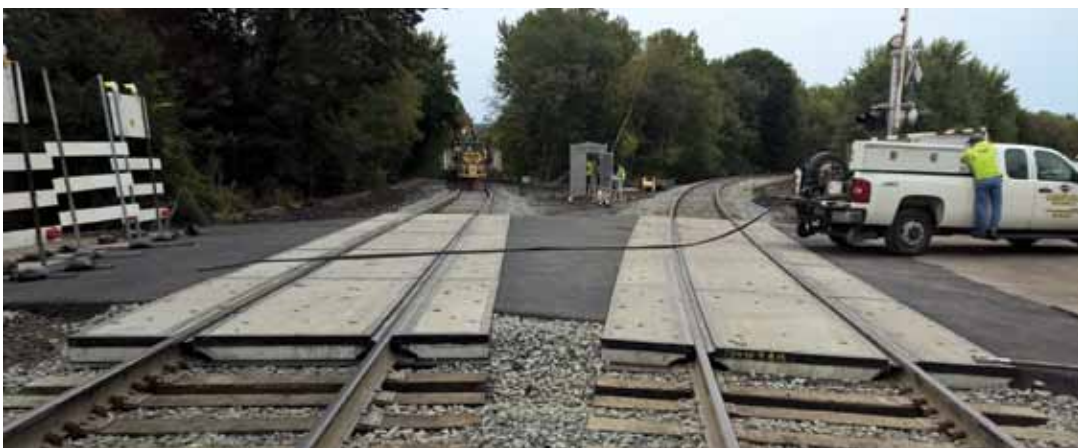
Newly installed concrete panel crossings at Foote Ave MP 1.91 on Susquehanna Branch and MP 0.01 on Dunmore RT.
