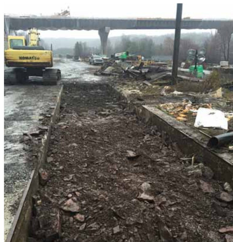
The new track bed through the pit area of the scale is almost finished for the track to be reinstalled for the runaround to be placed back in service.
