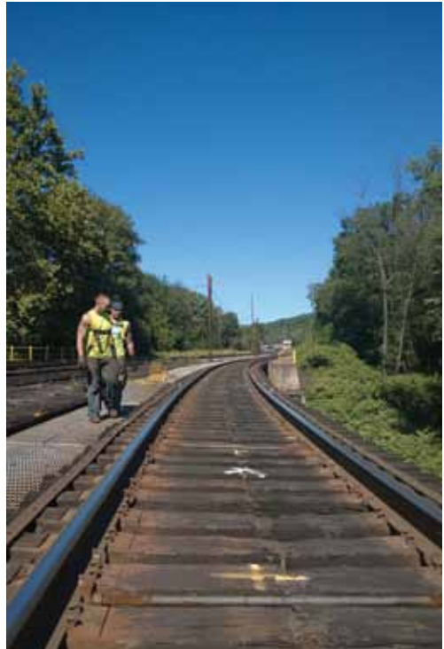
The middle of the Lackawanna Bridge from the view of the Susquehanna Branch with Matt Minnich and Aaron Cassel preparing to shim the bridge beams.
