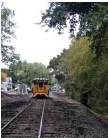
RBMN Mark IV running a pass on the Dunmore RT MP 0.02 relining the track to match the new location of the Duryea Jct Switch.
