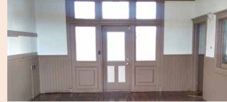
The main room in the Cressona Station as the building is being remodeled for the Signals Department.
