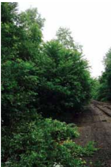
Brush close to the west side of the St. Clair Running track was pushed away to open up the ROW and keep the brush from hitting the trains.
