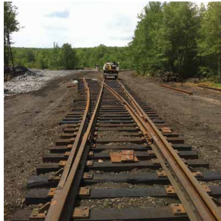
New switch installed on Ebervale Running Track just north of Ashmore Jct for Coal Contractors
