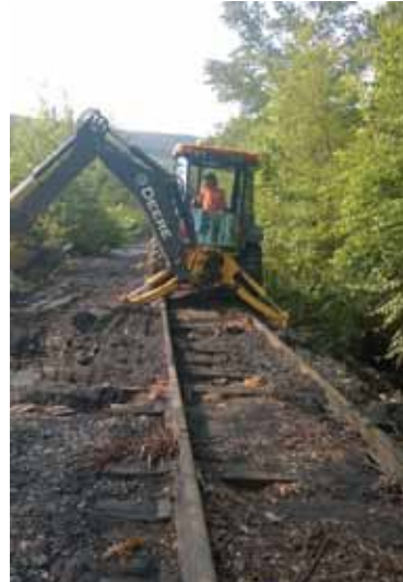
Brendle Stufflet operating the backhoe repairs a washout section on the track to restore the track to service.
