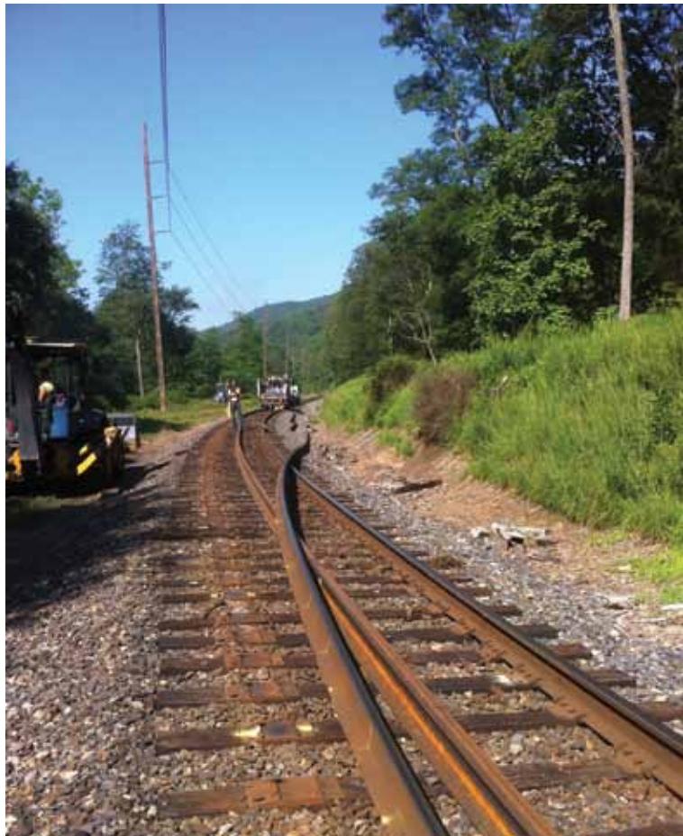
With the new rail string in the middle of the track, crews begin the process of removing the old rail from the high side of the curve to replace with the new rail string at MP 91.0 on the Reading ML.
