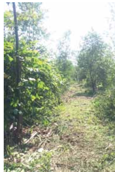
The rails are visibly clear after the first pass of brush cutting is performed on the Shenandoah Running track MP 3.9.
