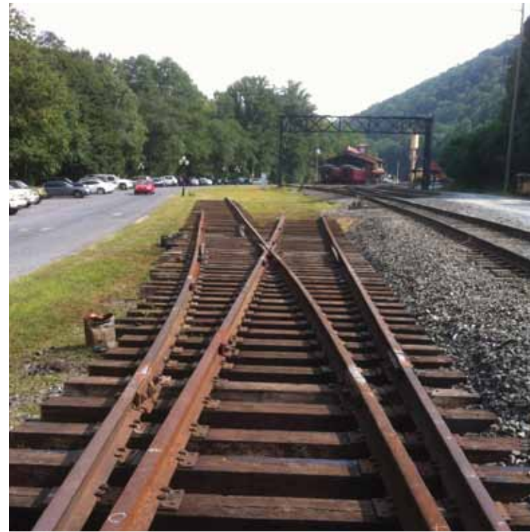
On the left is the new Car Shop Lead track, to the right is the second storage track in Port Clinton yard.
