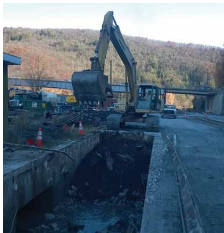
Scale is almost removed in Jim Thorpe yard for the pit to be prepared for suitable fill for the track bed and track to be reinstalled.
