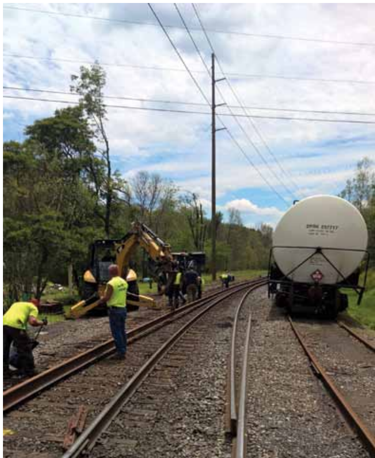
Using the backhoe to finish placing the new rail string on the Reading ML at MP 96.5, the gang jumps into action to begin securing the rail into its new home.
