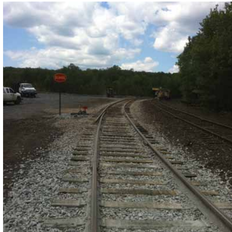
New Stockton Mine Siding on the Ebervale Running Track (formerly C&H branch north of Ashmore Jct) completed with split point derail.
