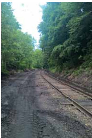
The brush was pushed far away from the west side of the St. Clair Running track around MP 0.3.
