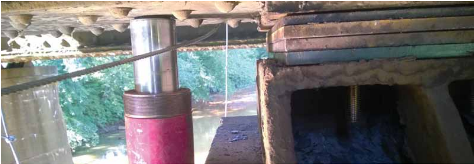
Using hydraulic jacks to lift the bridge beams for shim plates to restore the track geometry on the bridge over the Lackawanna River in Pittston.
