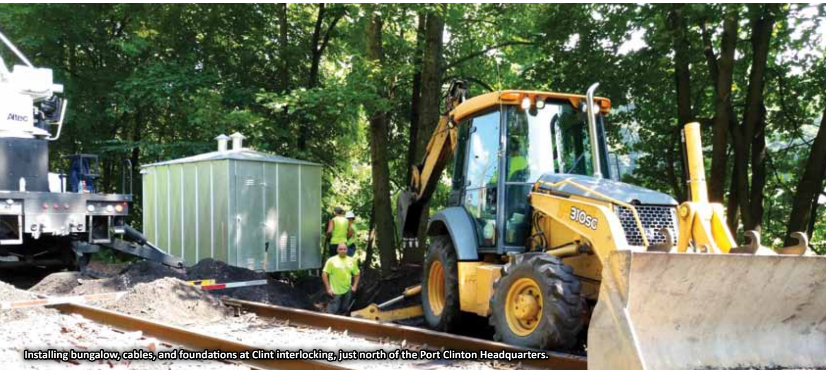
Communications Manager Matt Collins begins loading cable onto BT-2 to take to job site at Equilateral interlocking. Location was only accessible by rail, complicating installation.
