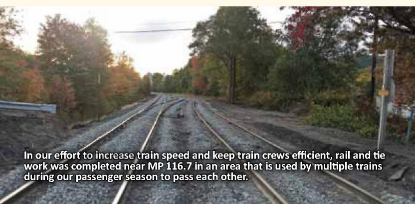
On our Main Line at MP 116.6, we dumped ballast after rail & tie work was completed. This was the last step needed on our way to increase train speeds.
