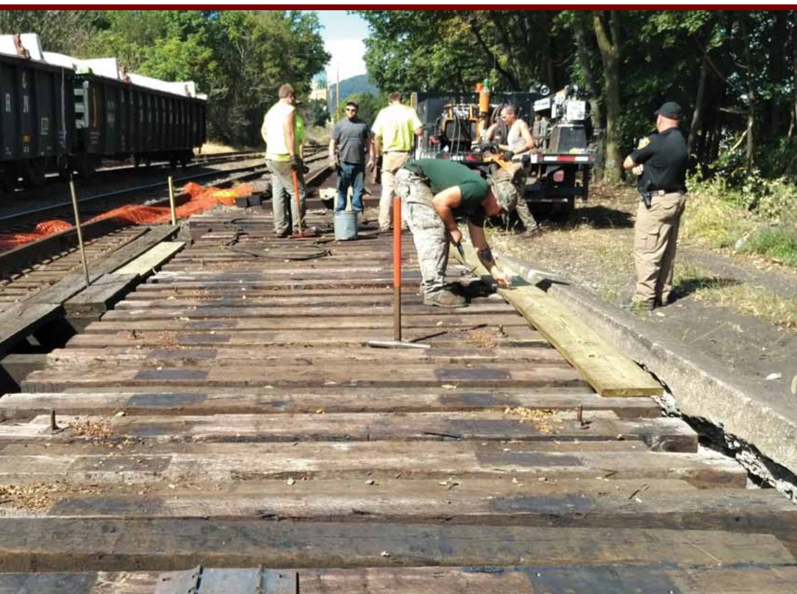
Matt Sloskey, Ben Cole, Dakota Reber, Eric Thompson, Brad Kunkle, Curt Williams are laying out and installing the track across the bridge. Officer Cromyack observes.
