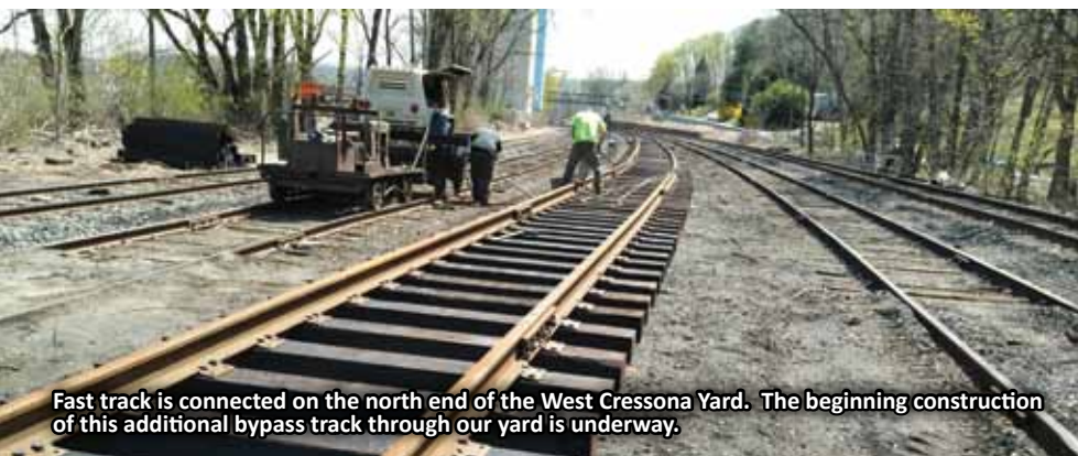
Contractor is replacing ties on track 2 MP 96.5 to start using the track to bypass trains in the lower Tamaqua Yard.
