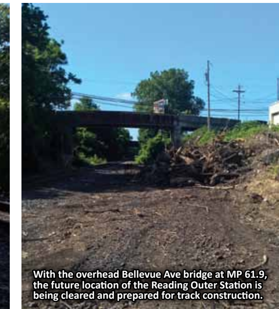
The future area for the Reading Outer Station MP 61.9 is cleared for the track construction and layout for the tower.
