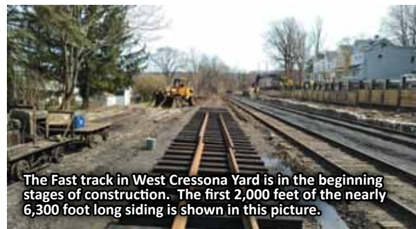
Dale Homm is busy clearing and laying the new switch for track 7 in North Reading Yard. This track will allow for additional classification of freight in the yard.
