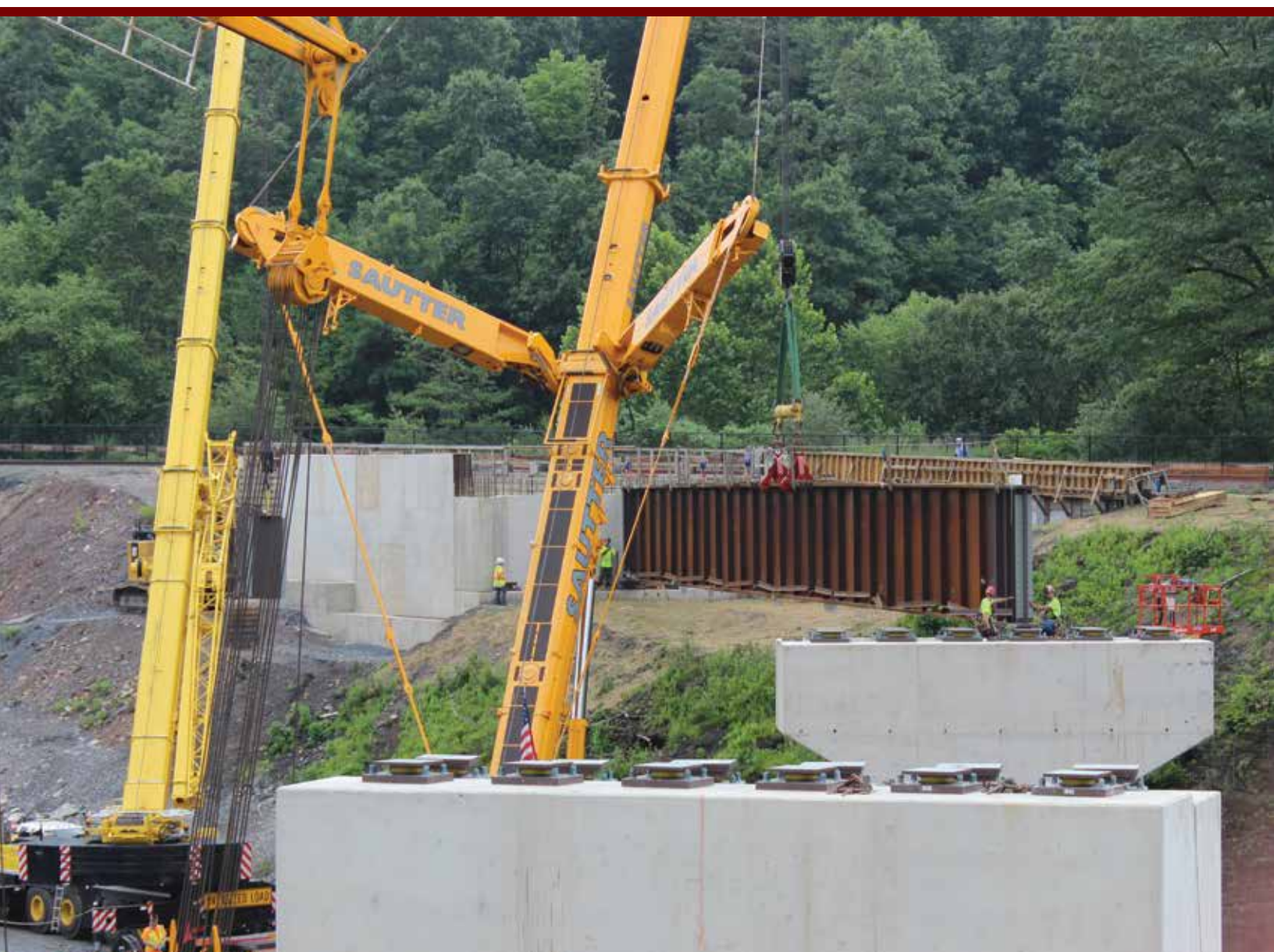
The first beam is set at the Nesquehoning Bridge on the morning of July 11, 2019.
