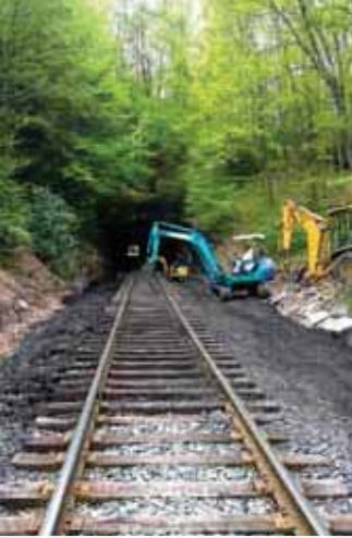
Work underway on the Tamaqua Tunnel MP 100 on the south portal to gain additional car clearance.
