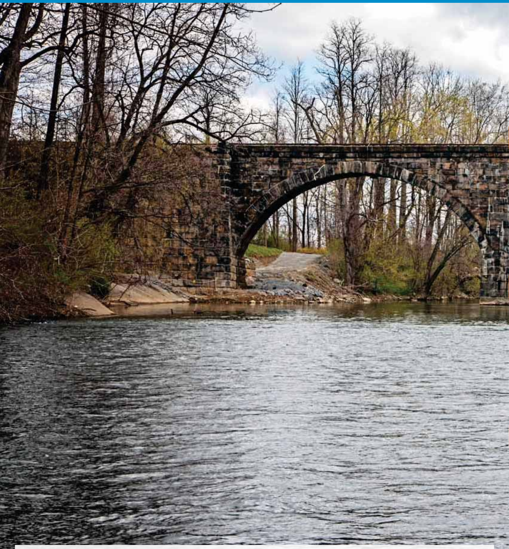
A view of the Maiden Creek Bridge located in Ontelauntee Township, Pennsylvania. Photo by: Roxanne Richardson
