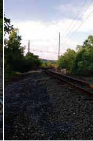
Curves recently gauged at MP 83.5 as part of the 10,000 feet of gauging to be completed this summer on the Reading Mainline between MP 81 – 90.
