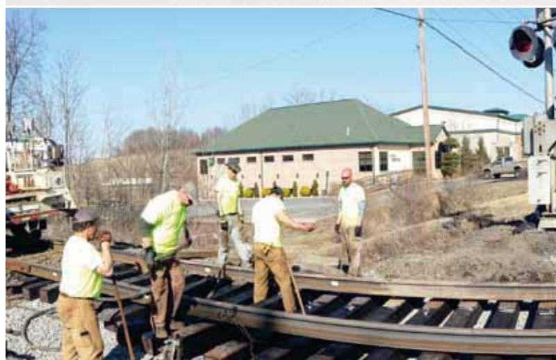
Reading and Northern gangs were all working on the crossing to get it done by the deadline of April 15th. Here, they installed new rails and spiked up the ties.
