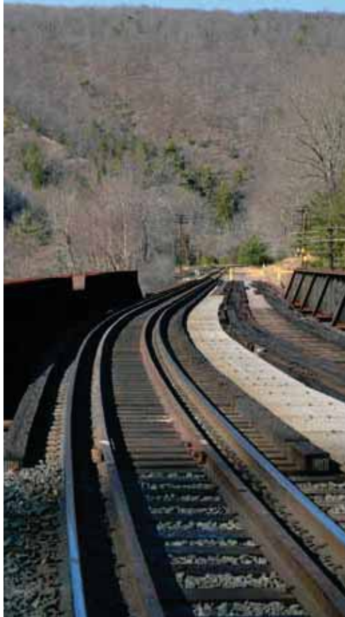
Bridge No. 130.90 deck replacement on mainline MP 130.9 north of Jim Thorpe, PA.
