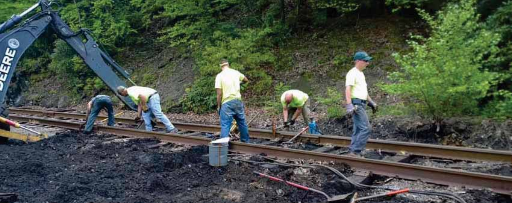
Maintenance gangs installing 1 of the many temporary crossing for bridge work this summer. This crossing is on the Saint Clair RT MP 0.2. From left to right John Brown, Duane Zimmerman, Matt Minnich, Larry Weller, Duane Engle
