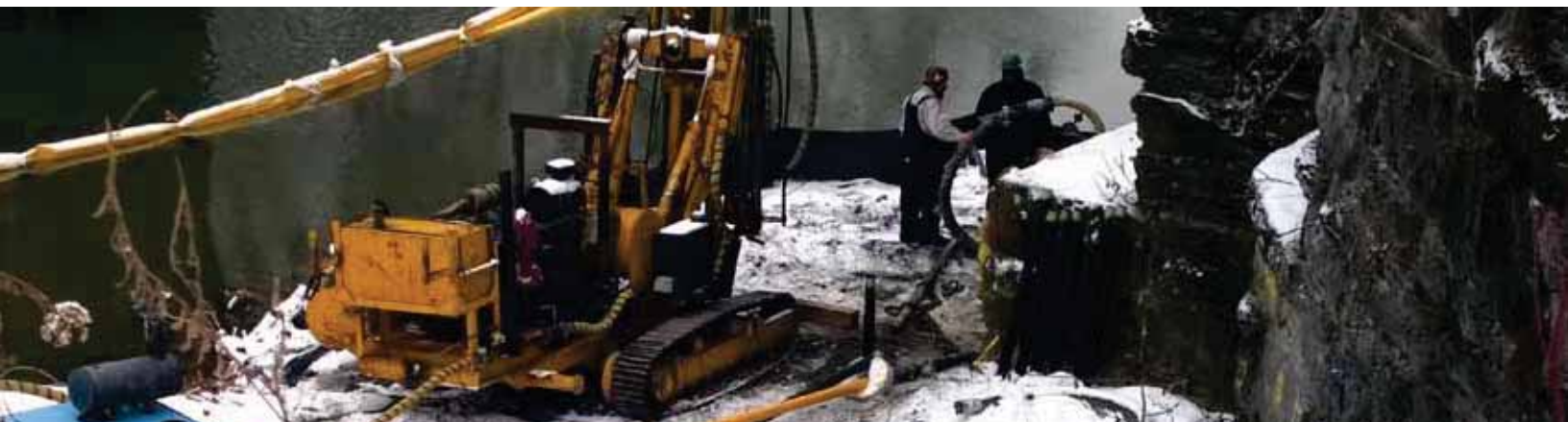
The men worked in freezing temperatures and snow to solidify the area under the structure. Here, they are drilling holes and pumping concrete under the abutment to make a strong base.
