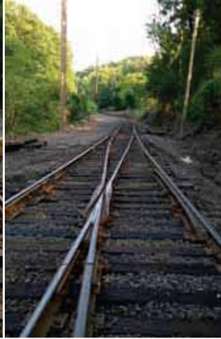
Recently rehabilitated switch at MP 75.2 as part of the Mainline switches getting a face lift this work season.
