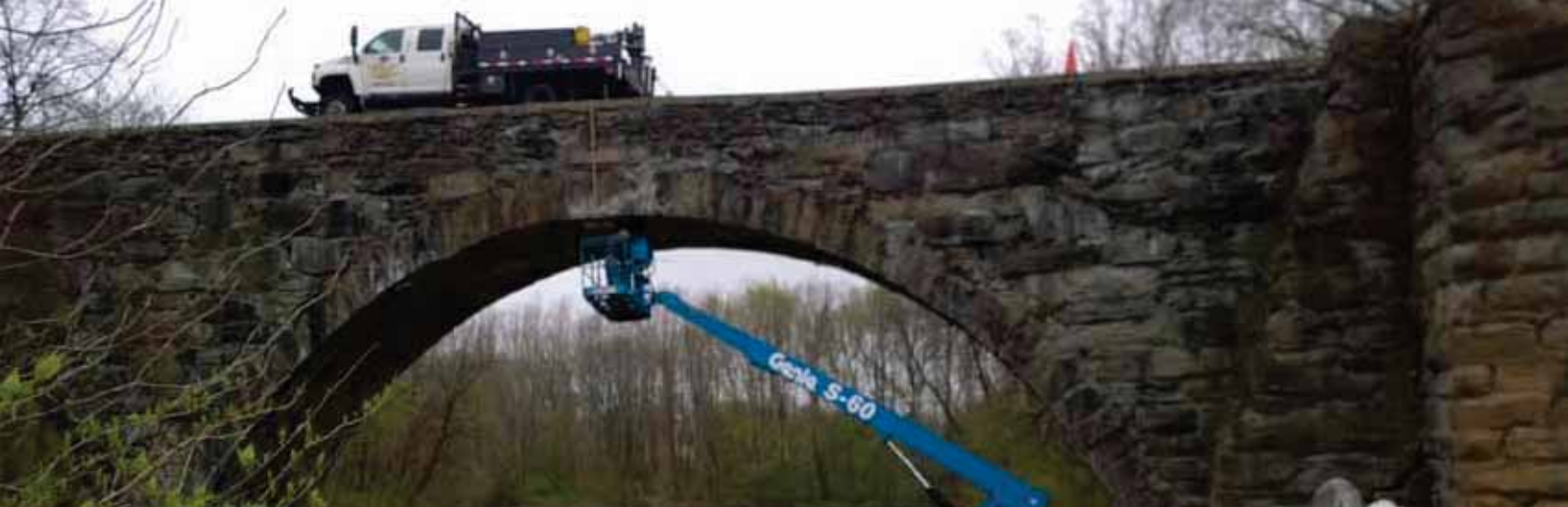
The bridge crew used a man lift to get up to the arch and hand pump grout into the cracks and point the stones while MOW was raising and lining the track up top.
