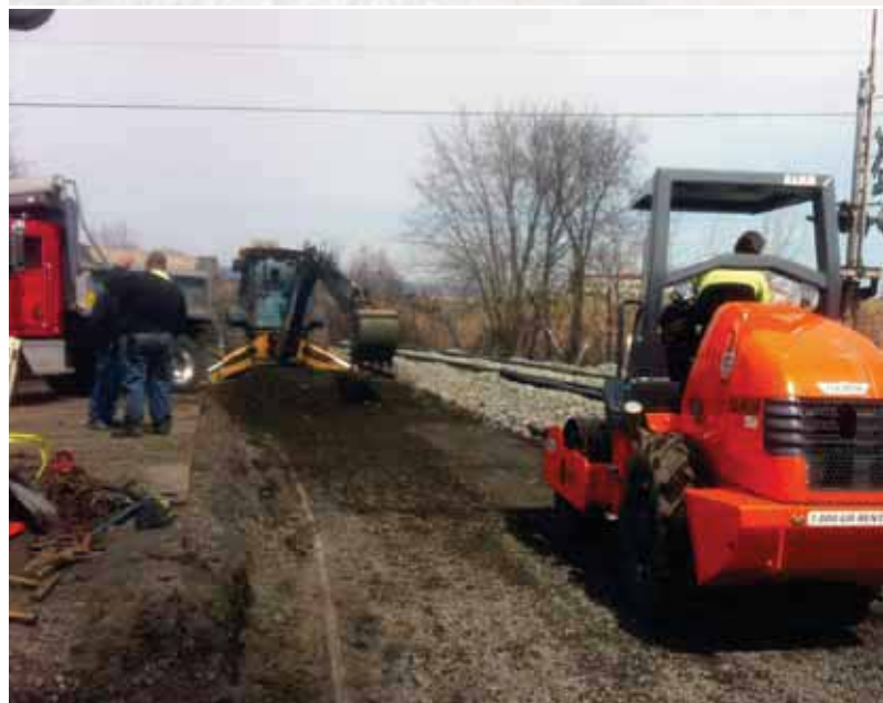
Here, the guys are digging out the old crossing and rolling it to compact the base layer for the new crossing.
