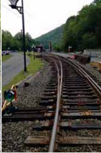
Work underway on the three new switches being installed at the Port Clinton headquarters MP 78.4.
