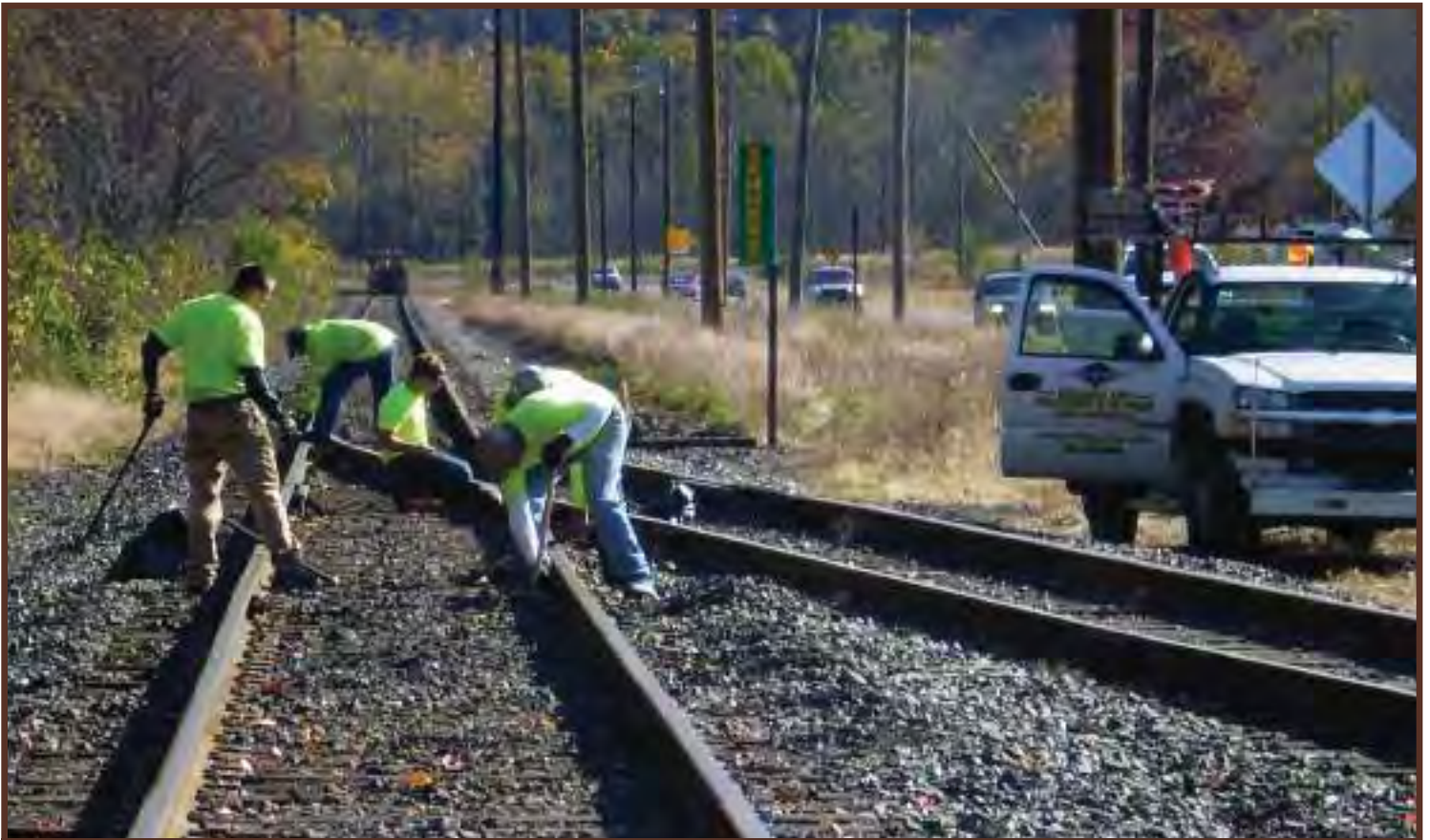
Multiple departments working together on the installation of the Wildcat Road Crossings.
