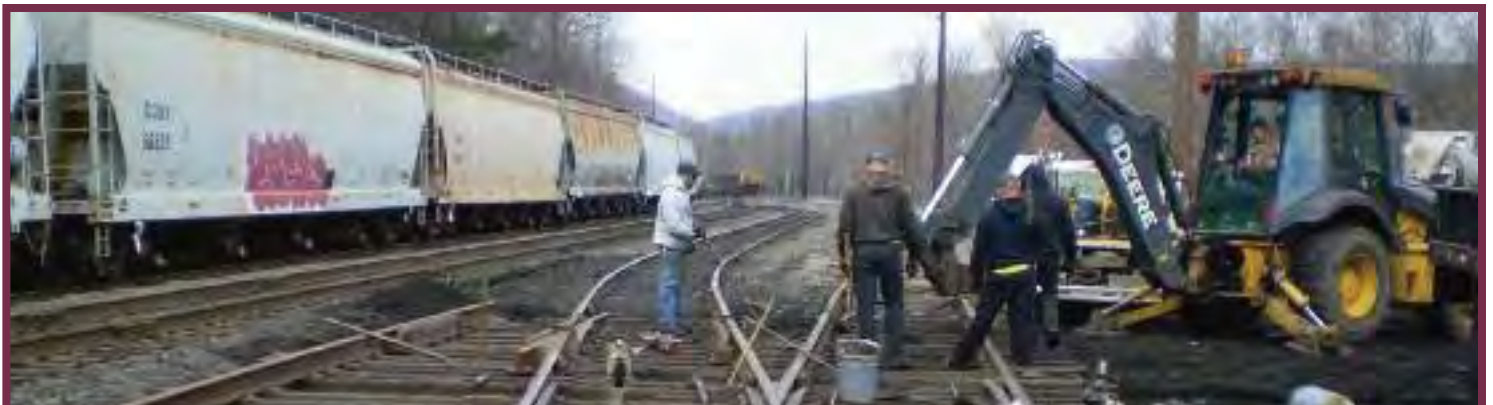
(L-R) John Brown, Mario DeMarco, Chris Nefos, Larry Weller & Dale Homm rebuilding #3 switch in the Tamaqua Yard.
