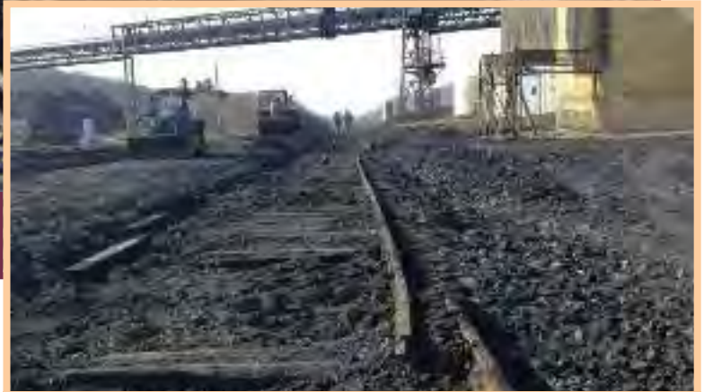
Dale Homm's excavation work at Gilberton Coal Company uncovered track that has been buried for over 25 years at the exact location a new siding was needed for new outbound coal business.
