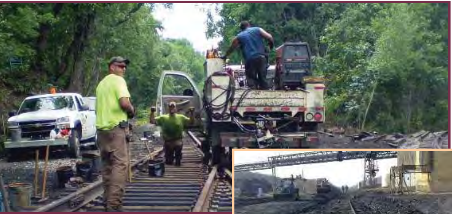
(L-R) Jason Witner, Shawn Slusser, Ryan Rupprecht (flexing) & Jose Mendoza constructing the south switch for the Scranton Runaround extension.
