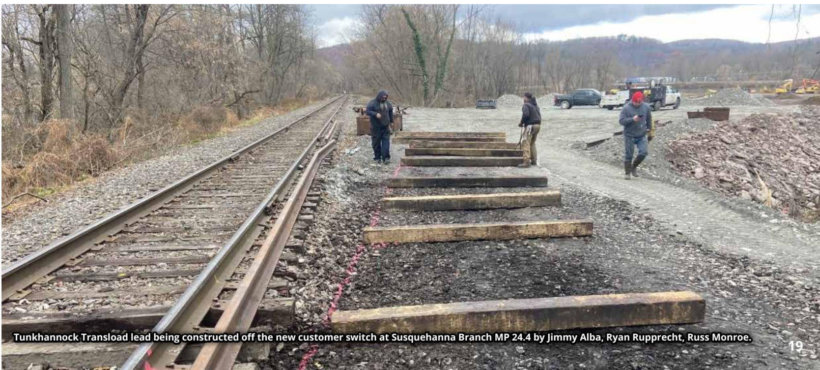
Shawn Himmelberger, Aaron Cassel, Dave Hutton plating and spiking new timbers at the White Birch Road crossing in the Humboldt Industrial Park.
