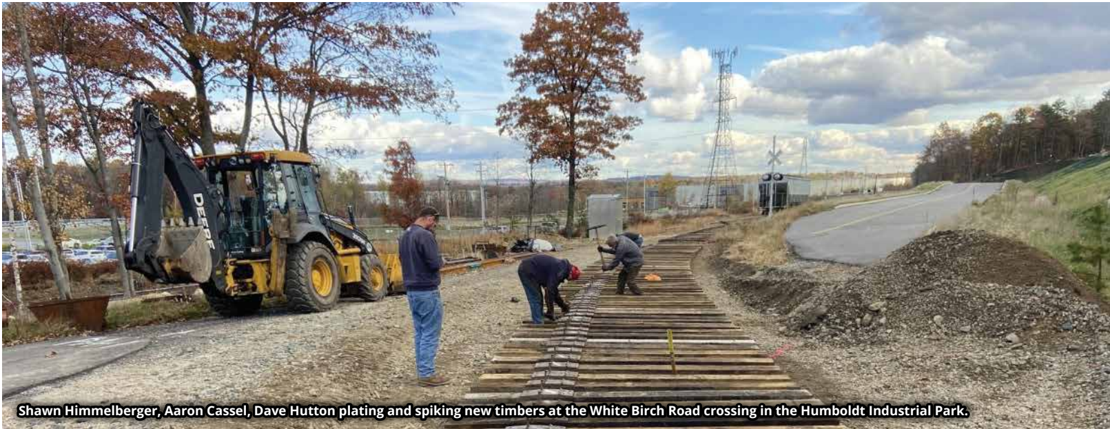
New 136RE rail string being installed to remove older 100lb rail at ML MP 108.6 by Dale Homm, Russ Monroe, Dave Hutton, Ryan Rupprecht.
