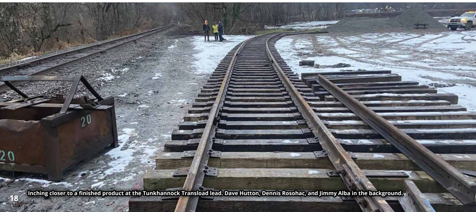
Tunkhannock Transload switch being constructed off the Susquehanna Branch by Alex Scubelek Jr., Shawn Slusser, Russ Monroe, Ryan Rupprecht, Jimmy Alba at MP 24.4.
