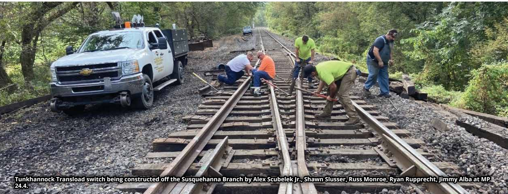
Plates being laid for new rail by Abe Kemmerer, Blake Handling, Dennis Roshac, Silas Bausher on Hazleton Line MP 115.
