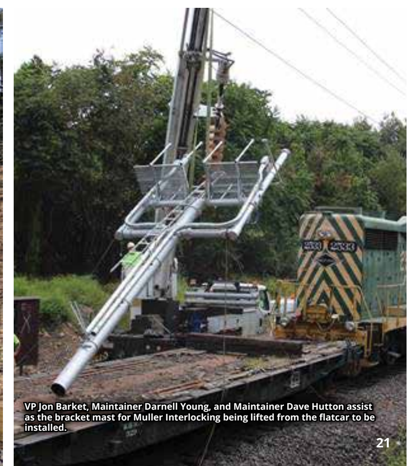
Three folks from the Car Shop are involved in the set up and welding of the signal post; John Dubick (left), Jim Sommers (on ladder) and John Byassee. In the upper right hand side Maintainer Darnell Young is one of two people holding rope to keep the proper alignment of the post between the time it was set in the foundation until it was welded into place.
