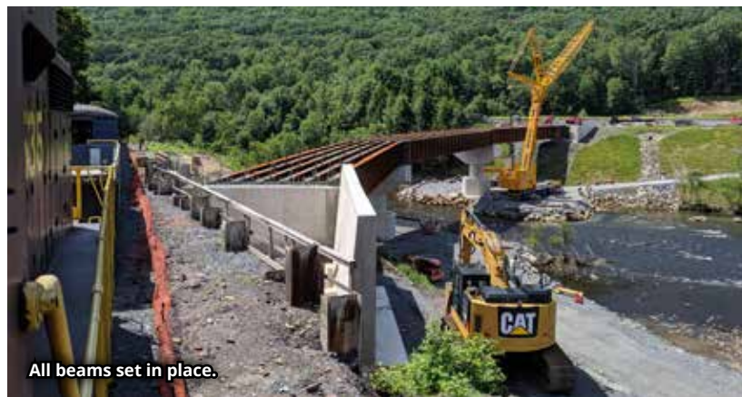
Railing in place for workers to apply deck pans between the beams.
