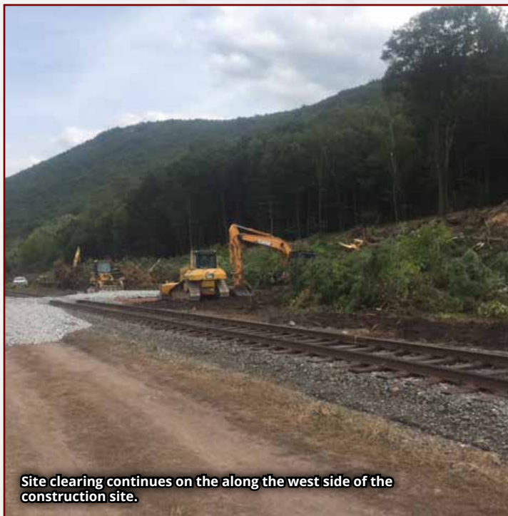
JD Eckman, the construction company who was awarded the bid to build the bridge, struck ground on August 14, 2017 to begin clearing the area for construction. Phase I Lehigh River bridge is seen in the background.
