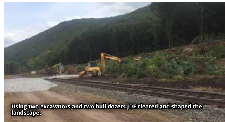
JDE brought in large excavators to clear the landscape. First, removed all trees and shrubs.
