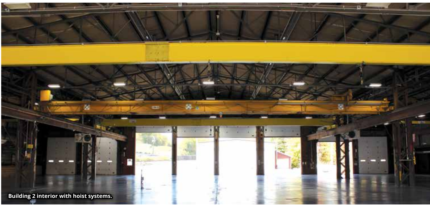
Building 2 interior with hoist systems.
