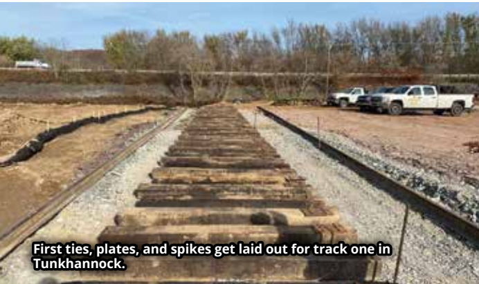
Switch grading complete and ready for construction at the Tunkhannock Sand Facility.
