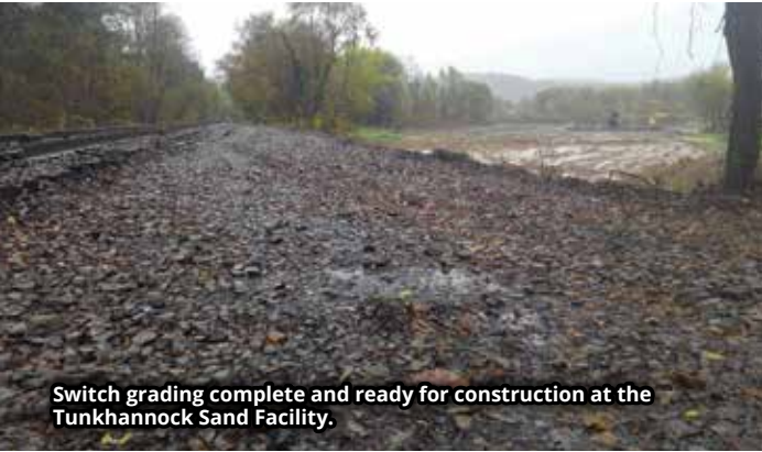
Early stages of the Tunkhannock Sand Facility can be seen with the beginnings of site grading by Alex. Scubelek, Jr.
