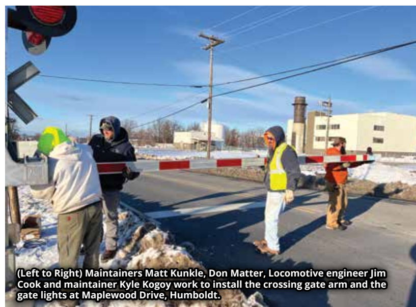
Locomotive engineer Jim Cook, working with the signal department to install the Maplewood Drive crossing gates.
