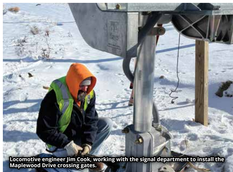
Electrician Ryan Boyer (left) and maintainer Don Matter (right) work to install cable at Maplewood Drive, with MOW working on the crossing in the background.
